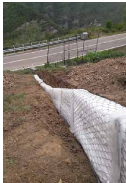
Backwater drainage for protection of road surface - Ottone (PC)
