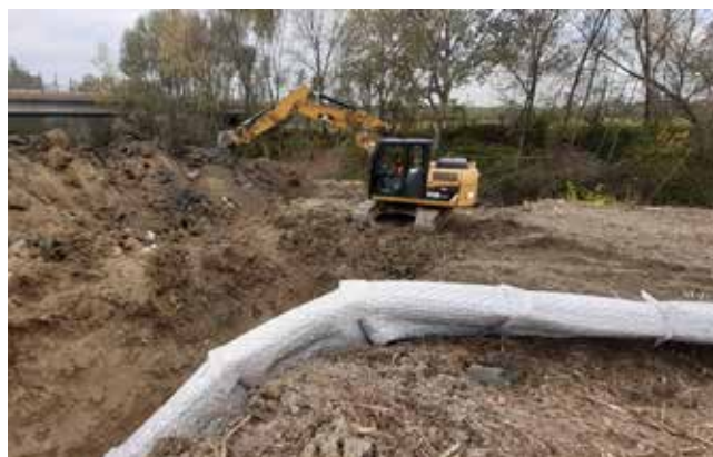
Drain in restoration of riverbed landslide, in detail the elevated one flexibility of modules - Cesena
