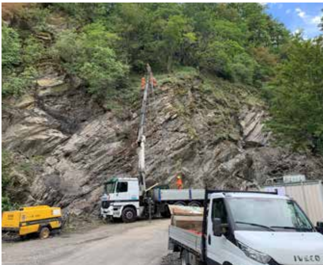
Pre-intervention unstable rocky slope - Fopla di Solignano (PR)
