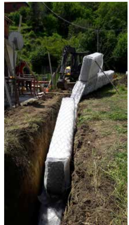
Drenar foundation protection in confined spaces with draining chimney and sheath - Tresana (MS)
