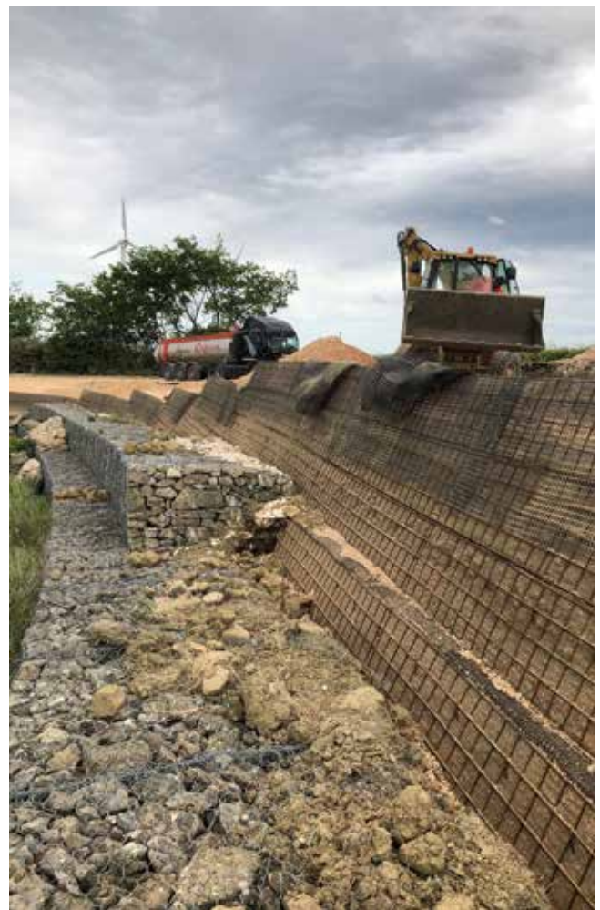
Mixed work with gabion base and top in soil reinforcement -Acerenza (PZ)
