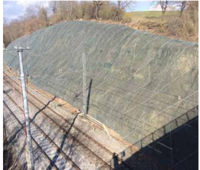
ArrPet, stabilization of the railway slope with very fine soil - Orte area (VT)
