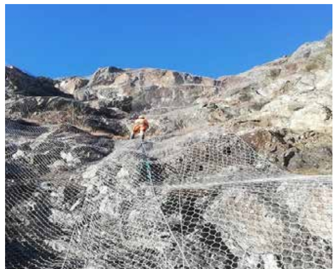
ArrFort strengthened rock fall net protection - Val d'Ossola (VB)
