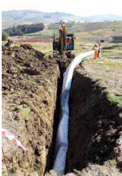
Drenar is installed continuously in pushing soils Vulturara Appula photovoltaic field (FG)
