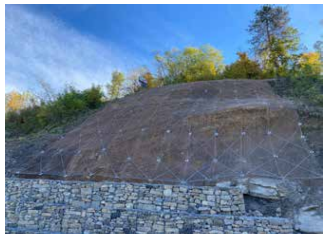
Arco system, road under-slope stabilization in loose ground, with gabion at the foot - Ferriere (PC)
