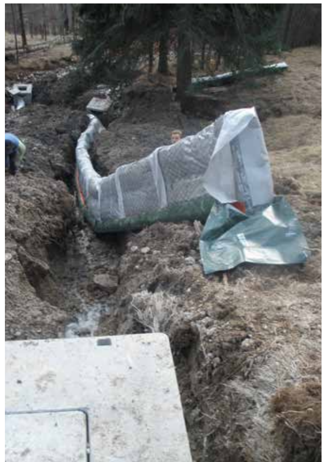
Installation in a forest area that is difficult to access - Selva di Cadore (BI)
