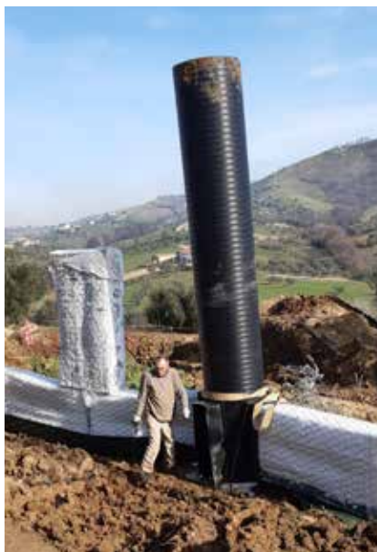
Graft Drenar with sheath and draining chimneys in prefabricated well outside excavation - Tortoreto (TE)
