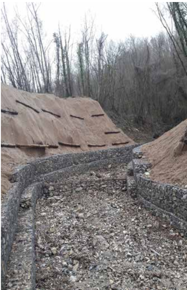
Hydraulic arrangement and slopes stabilization of low impact gabions and geocomposite Arco - Genoa
